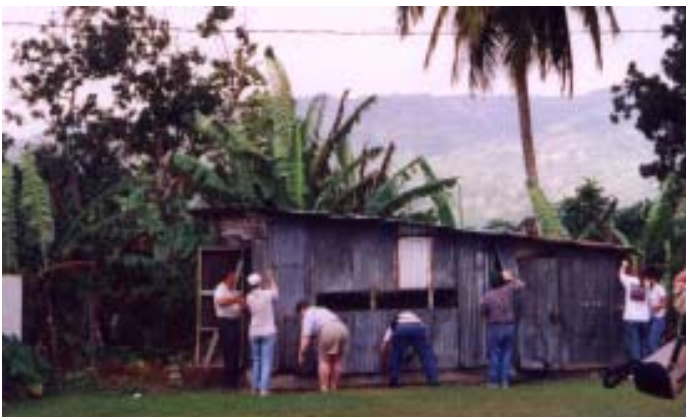
The Jamaica work team tears down the chicken coup at the Lyndale Girls Home. Some of the tin was salvaged and used for the new coup.
