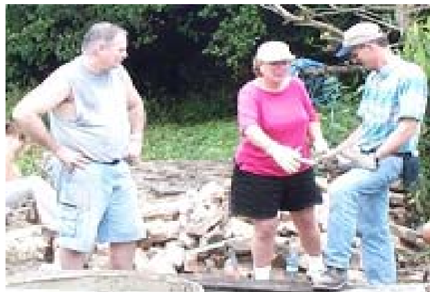
From left, Jerry Phillips, Lisa Baum-Waters and Paul Hemingway work at the construction site at the Chapel in Floro Perez, Cuba. Jerry's wife, Patti and Erwin Lopez also traveled to Cuba with the FUM Work Team.
